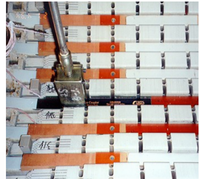
SSCS BEING INSTALLED ON A TURBOGENERATOR
