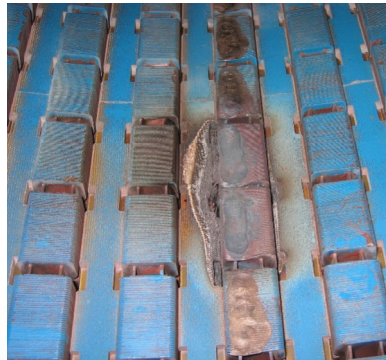
FAILED TURBOGENERATOR STATOR WINDING
