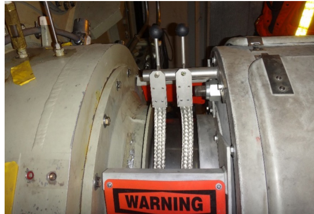
SHAFT GROUNDING BRUSHES ON A TURBOGENERATOR
